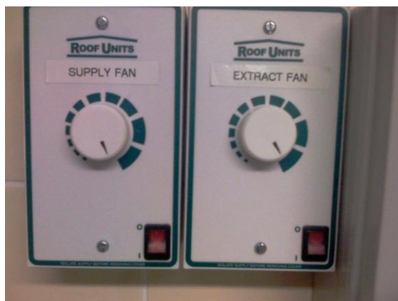
Fig 1 – Fan controls set at full speed
